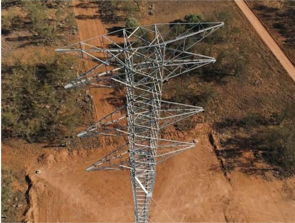
Transgrid's Legacy 100 workers will be rigging up new transmission towers and lines to connect the Victorian, NSW and South Australian energy grids. Picture: Supplied
