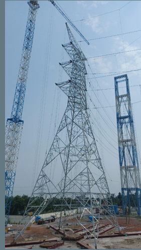
330 kV Heavy Angle Strain 64m tall and 56t
